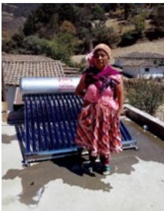
Installed solar panel, Estrellas Preciosas
